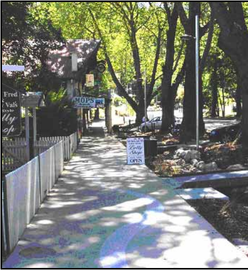
Lower section of Murchison Street, Marysville following the completion of Stage 1 works
