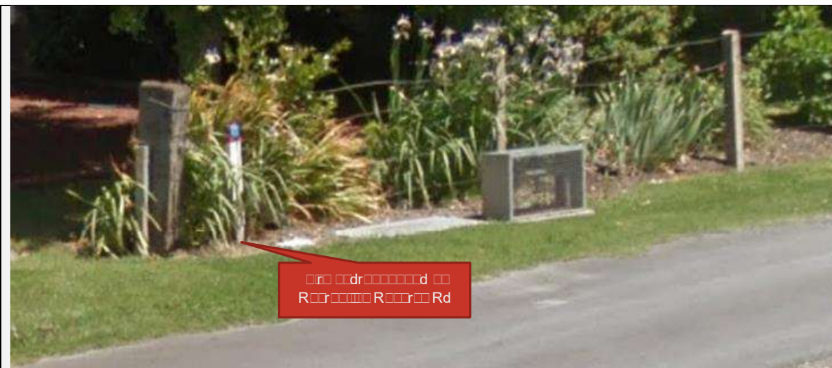
Photograph 12: Fire hydrant located within 120m of the subject site.
