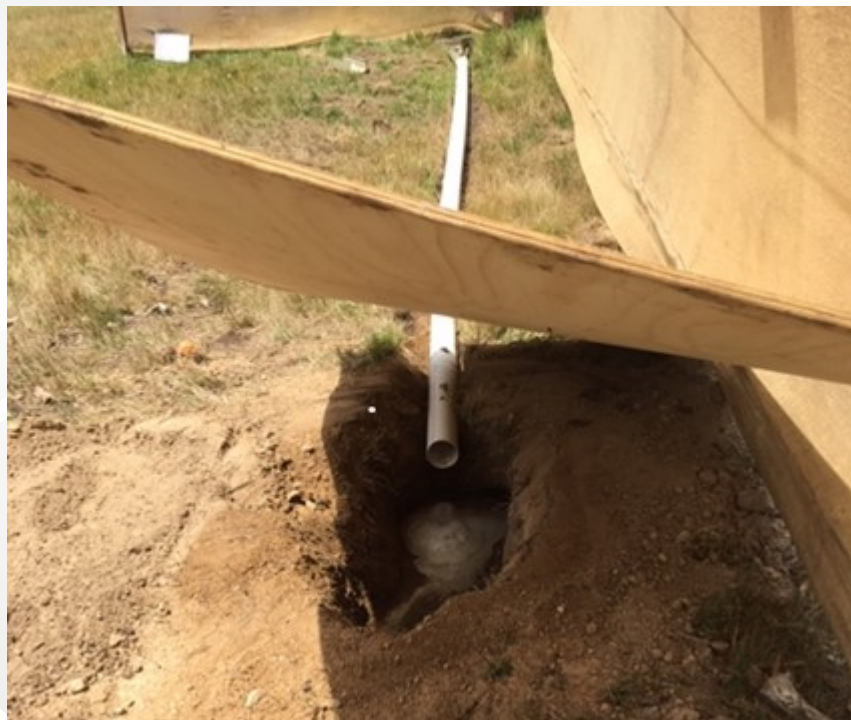
Figure 6: Urinal disposal pit
