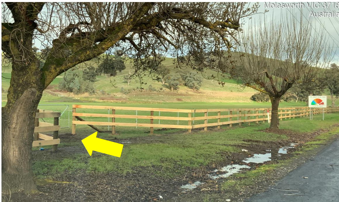
Photograph 1: Newly constructed access gate off Goulburn Valley Highway as per approved plans
