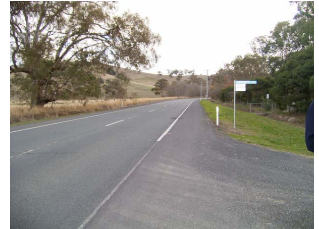
Photograph 5. The Goulburn Valley Highway in Molesworth is straight and clear, which is not conducive to lower travel speeds.
